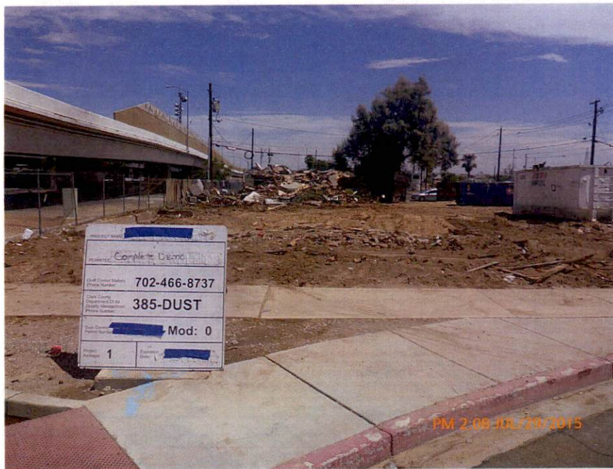
Photograph # 4 Alleged Violation # 1 View looking SE towards the footing of Building #2 (foreground) and Building #3 (background). The dumpsters are sitting where Building #1 once stood.
