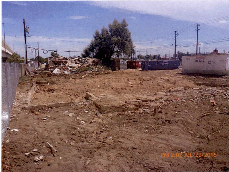
Photograph # 3 Alleged Violation # 1 View looking SE towards the footing of Building #2 (foreground) and Building #3 (background). The dumpsters are sitting where Building #1 once stood.
